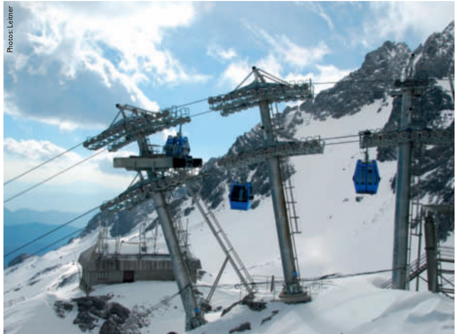
The three-piece tower before the upper terminal is required to handle the evacuation ropeway, with one of the two 6-passenger reversible evacuation cars parked on the lower tower.
