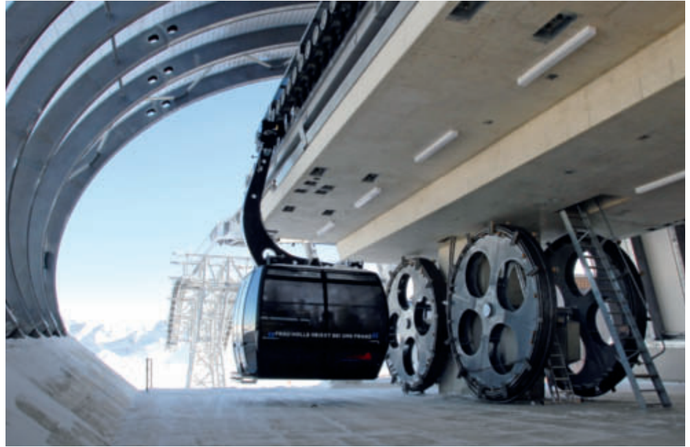
Incoming line to the top station of the 3S-Bahn
